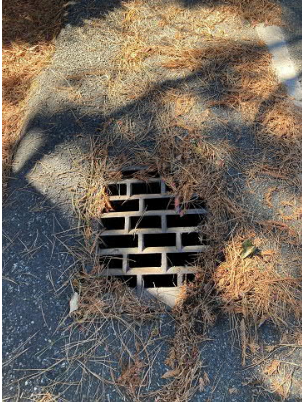
Picture 3: southernmost corner of Mercerwood Drive and SE 43 rd Place Following the mapped flowpath, this catch basin is across Mercerwood Drive.
